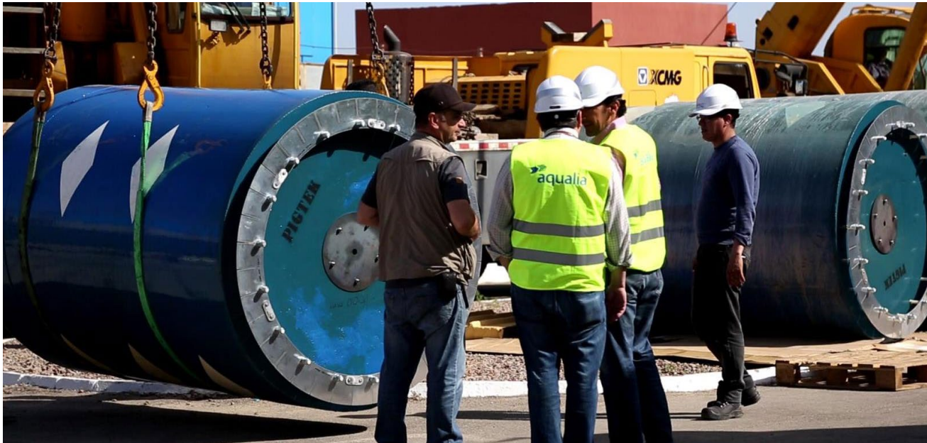
PIG technology applied for cleaning water intake conduits in the Mostaganem, Algeria, desalination plant.
