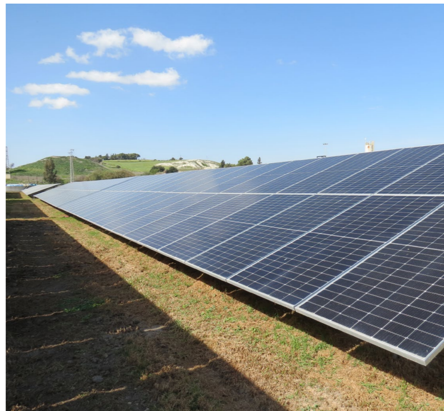
Solar panels installed at the WWTP in Jerez de la Frontera, Spain.
