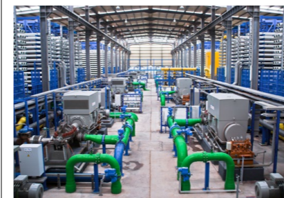
● Interior of the Mostaganem seawater desalination facility, Algeria.
