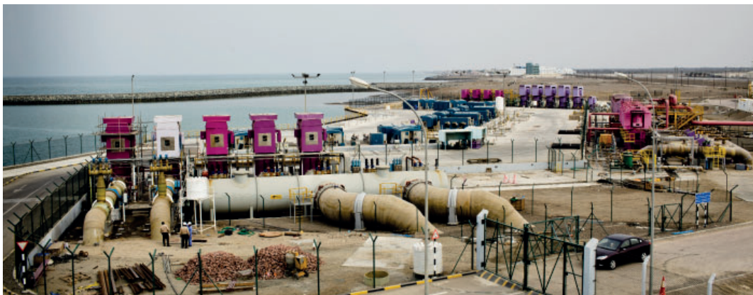
Seawater collection facilities in the port area of Sohar (Oman)
