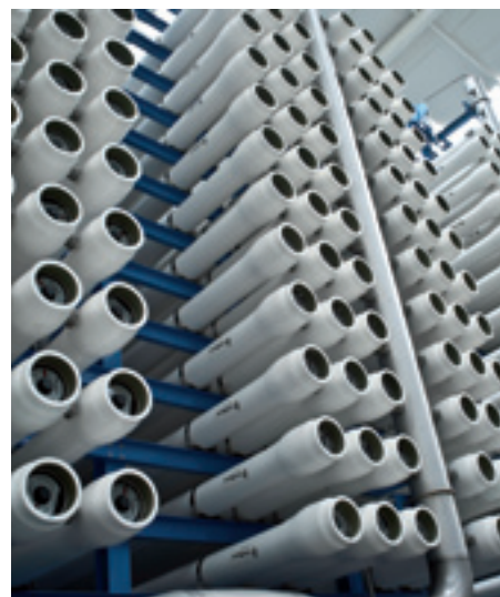
Membrane frame at Cap Djinet desalination plant.
