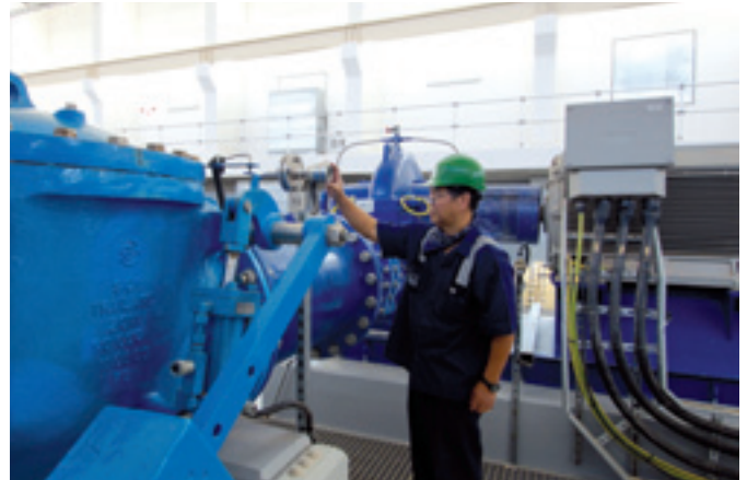
Pumping station of Al Ain, United Arab Emirates.
