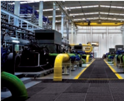
The aqualia Infraestructuras Cap Djinet desalination plant, Algeria.
