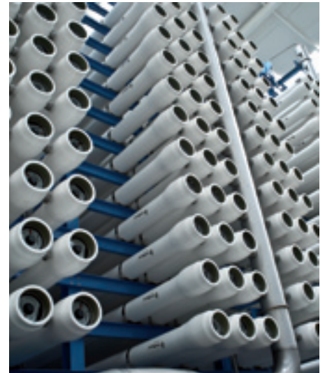
Membrane frame at Cap Djinet desalination plant.
