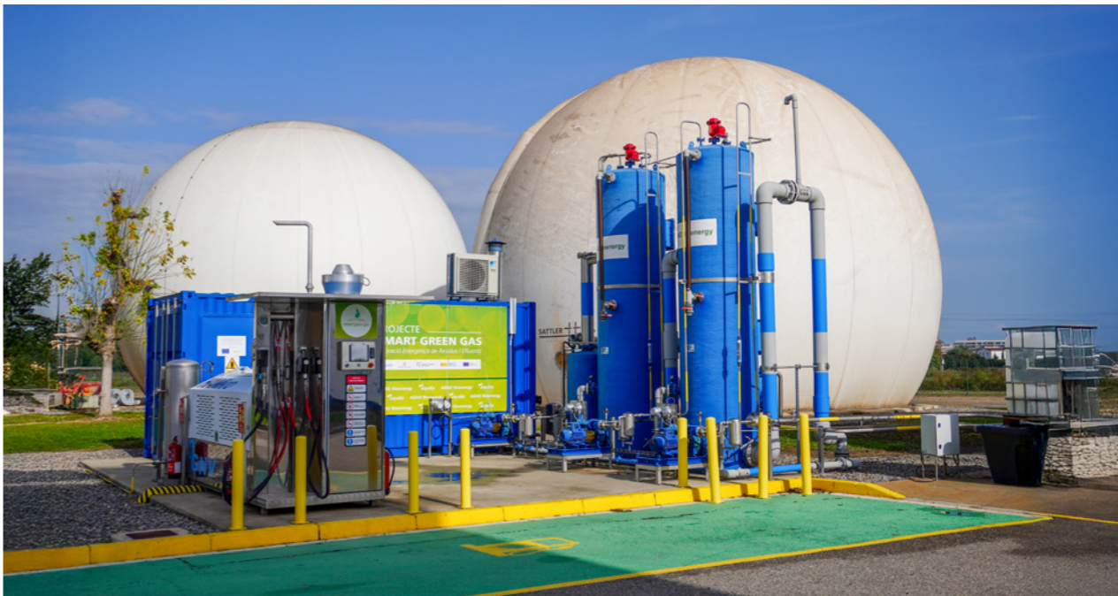
Wastewater Treatment Plant (WWTP) in Lleida (Spain).
