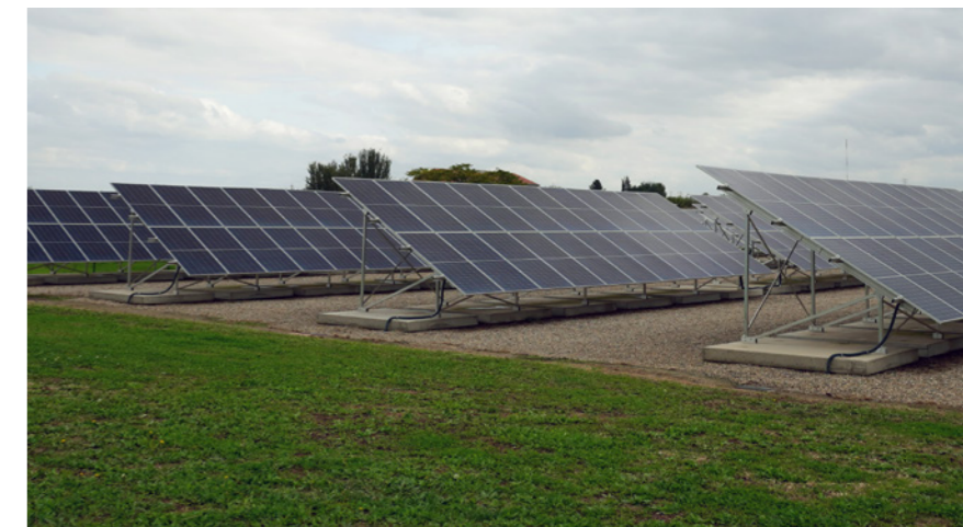
Wastewater Treatment Plant (WWTP) in Lleida (Spain).
