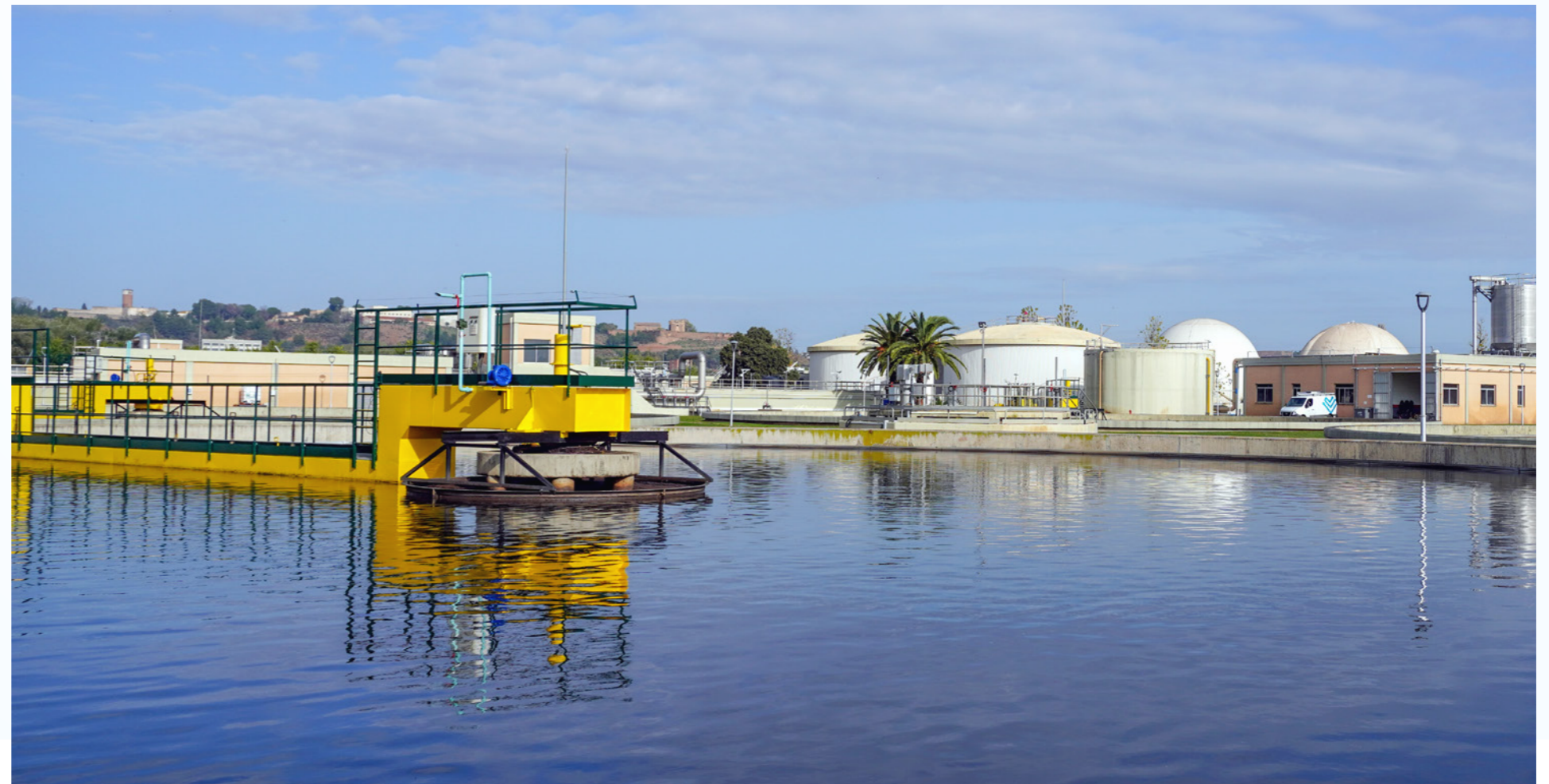
Wastewater Treatment Plant (WWTP) in Lleida (Spain).
