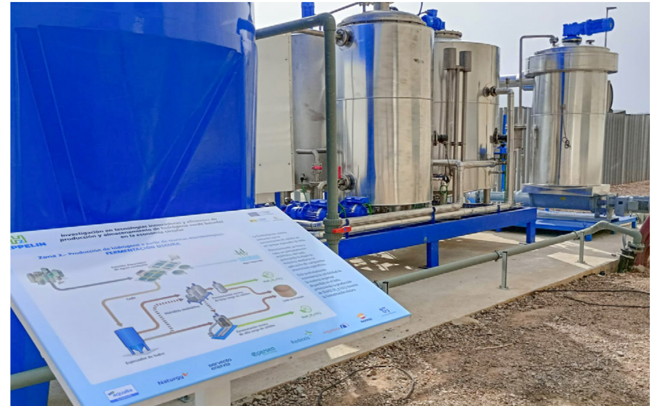
Wastewater Treatment Plant (WWTP) Isla Verde de Algeciras (Spain).
